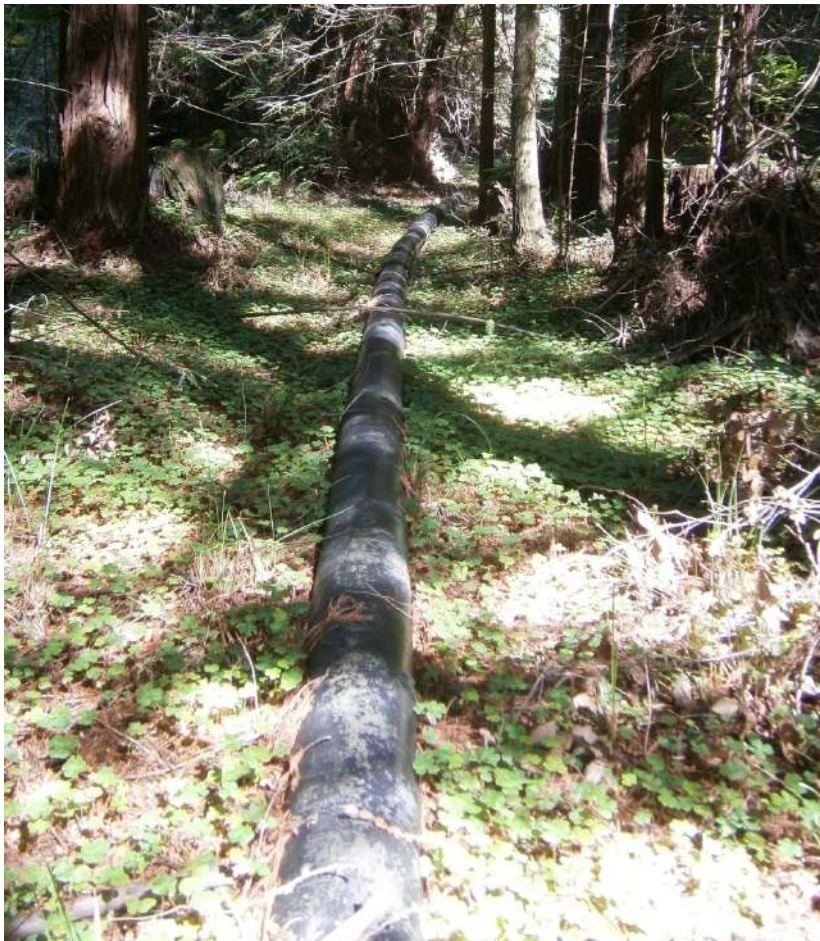
Photo: An aboveground pipeline on the Coast Dairies Property supplies water for the City of Santa Cruz.
